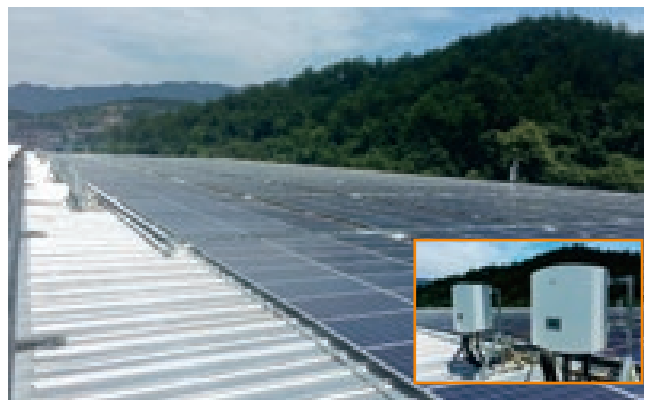
Hainan JiuLongGlass 1.7MW
