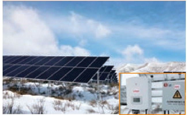
Shanxi Guangling PV plant 1.47MW
