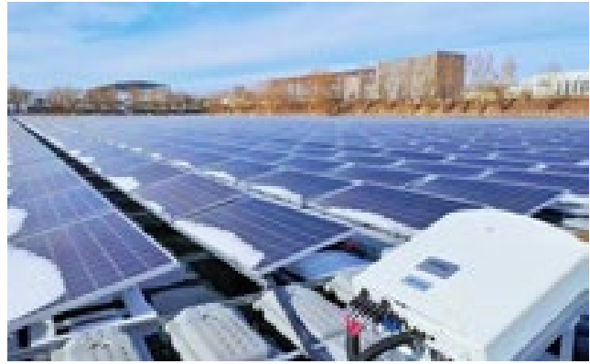
Beijing Shunzhen Green Harbor's Plant 5.5MW
