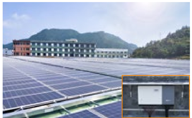
Tyco Electric, Panan Jinhua Zhejiang 1.5MW
