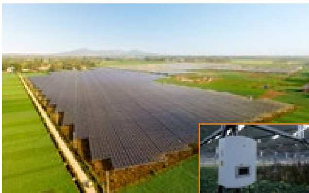
Hubei Guanyin Agricultural-photovoltaic hybrid PV plant 20MW
