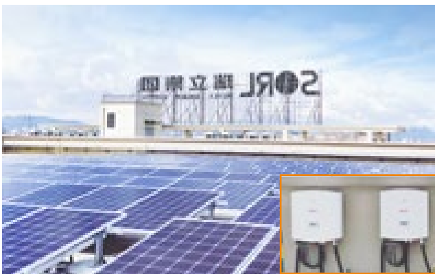
Zhejiang SORJ 3.9MW
