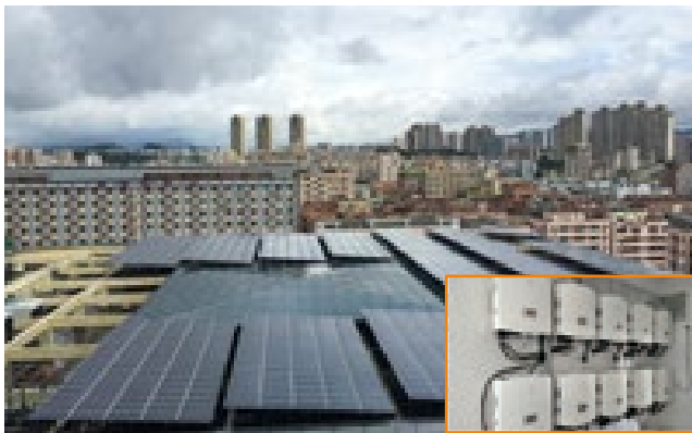
Shenzhen Jiangnan Times Building 600kW
