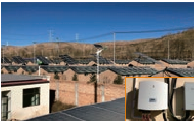
Qinghai HuzhuBanyan poverty alleviation PV Plant 2MW
