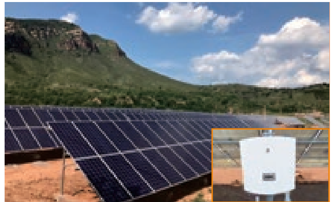
Shanxi Xiyang poverty alleviation PV Plant 7.2MW
