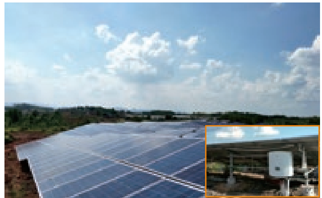
Jiangxi Ganzhou PV Plant 3.5MW
