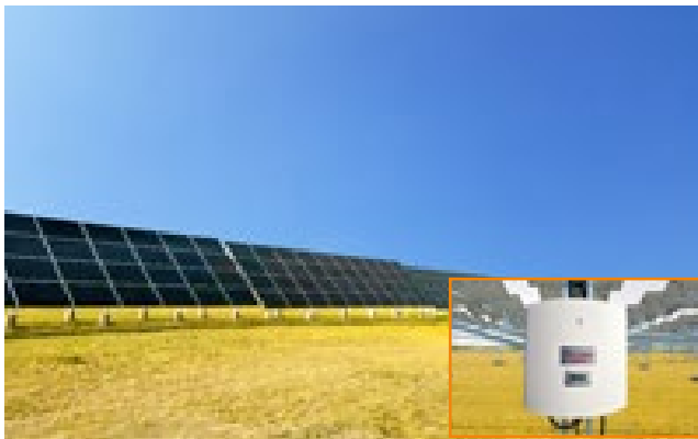
Huaneng Yimin surface mine PV plant 20MW
